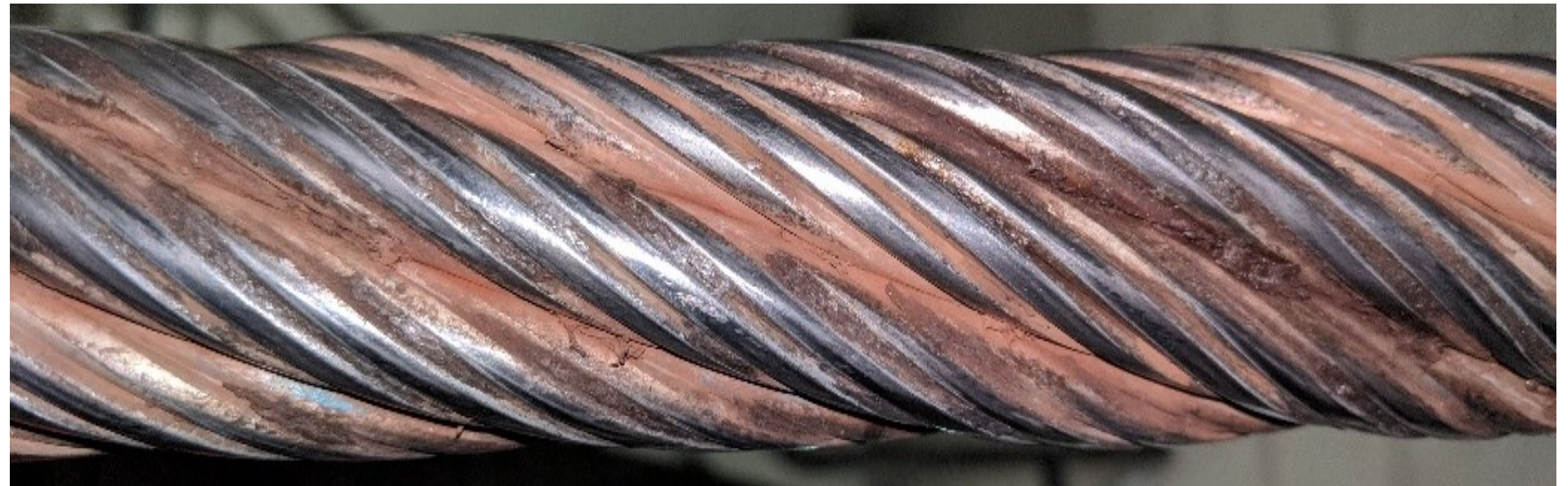
Corrosion induced by friction between touching strands
