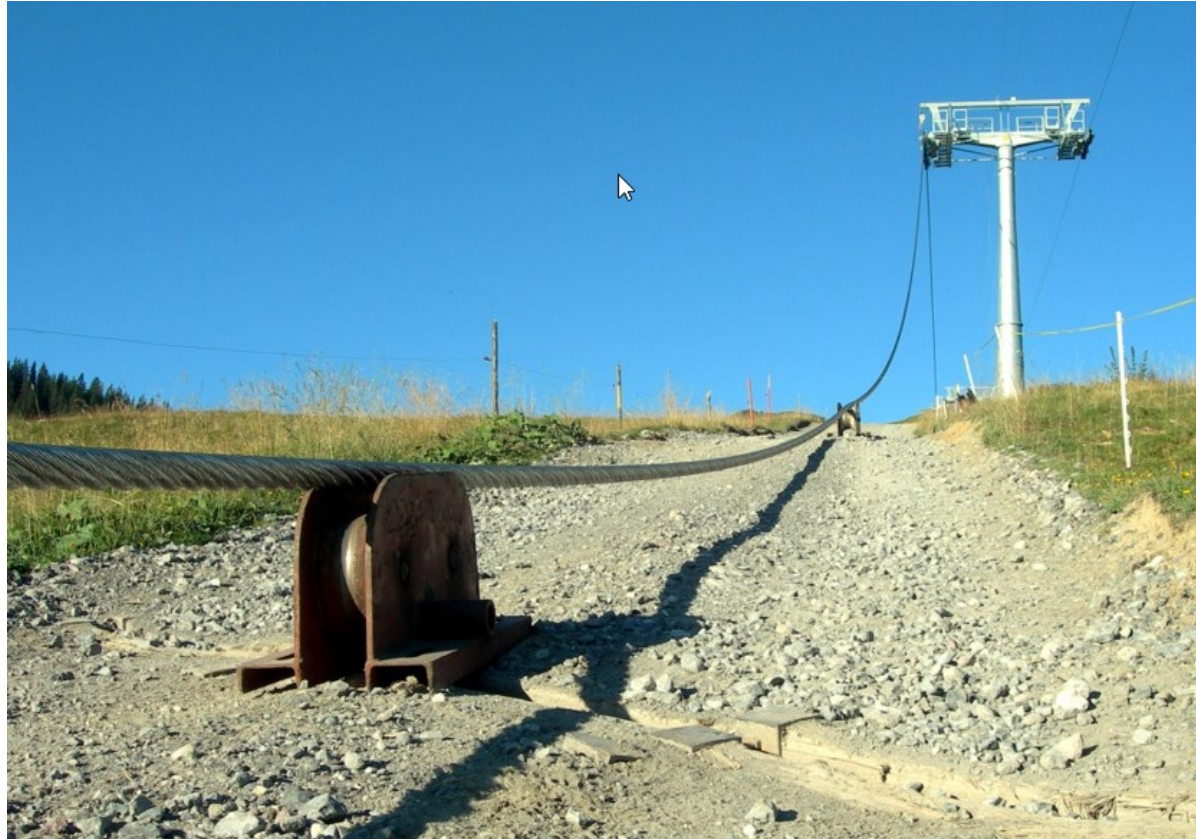
Abrasion - critical situation, rope too close to the soil
